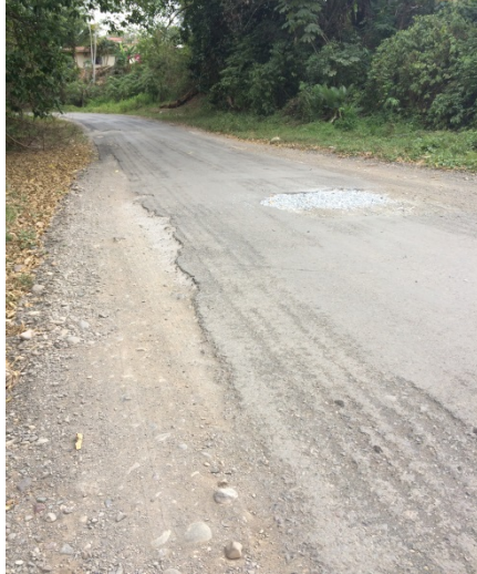
Condition of the highway to Esterillos Oeste
