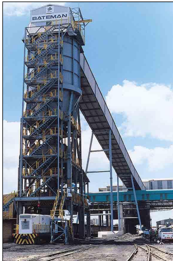
Figure 6.12 Station de chargement typique
