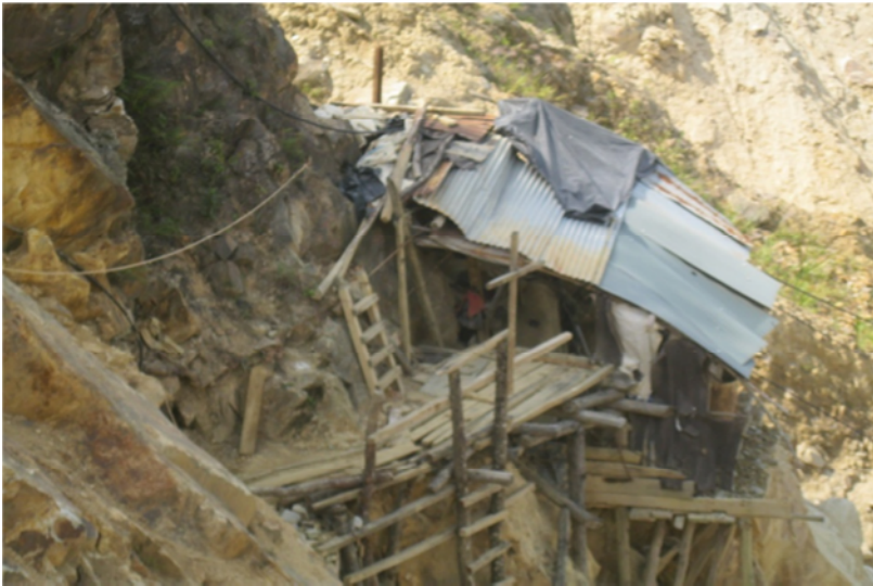
Figure 6. The illegal mine at Mina Esperanza, located within GCG mining title 147-98M in the Marmato region, was created out of roughshod materials and contains no safety features to protect workers.
