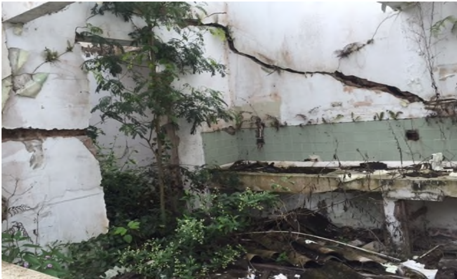
Figure 3. Severe infrastructure problems in the local hospital in Segovia were primarily caused by underground illegal mining.
